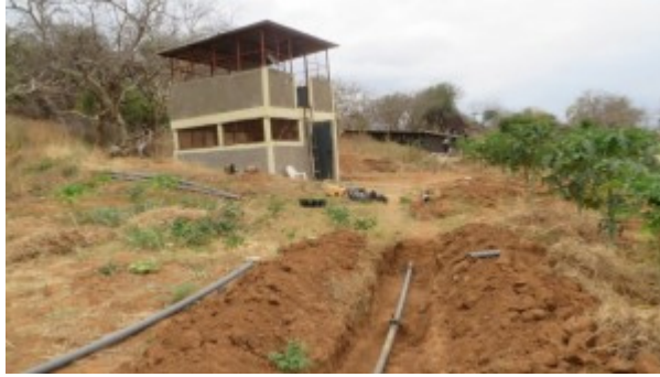
gate valve connection and regulate water flow from pan 1 to the tanks and also to and from pan 1 and 2
