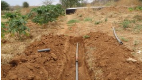
gate valve regulating water to adn from pan 1 and 2
