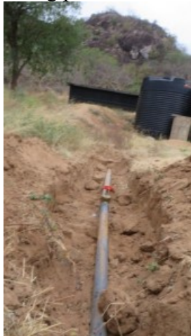
gate valve regulating water flow from pan 2 to the tank for irrigation
