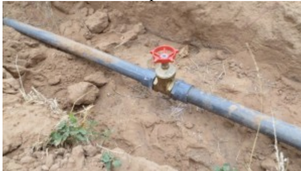
gate valve regulatng pan 2 to the 4 irrigation tanks
