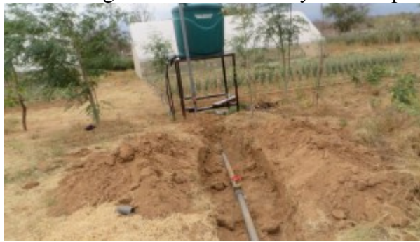
gate valve near tanks no. 4 at green house no.4 this complet the set of connection from both pan 1 and pan 2
